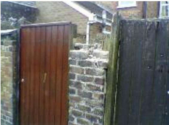
Before: Crumbling Walls
